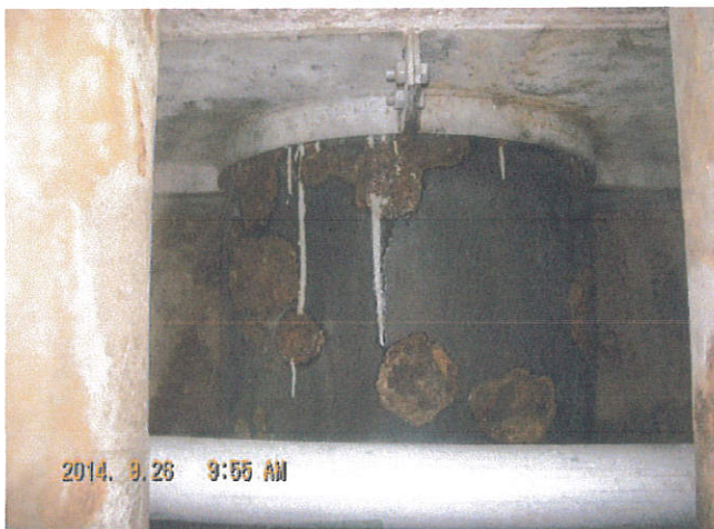
③Carry out descaling with a brush or spatula. Uneven rust and corroded spots can be observed.
