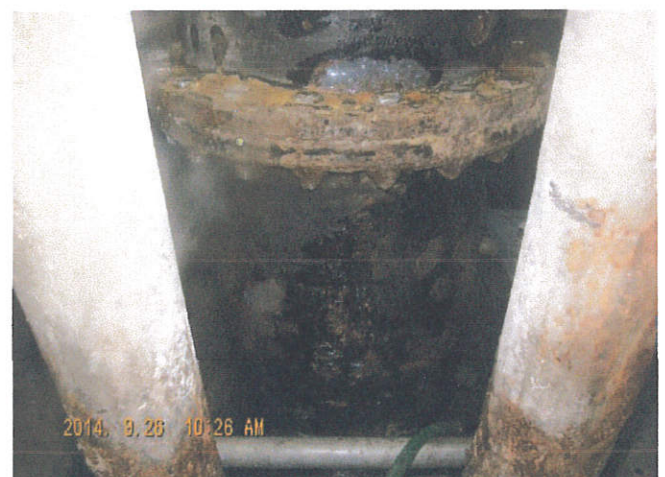
⑥ Then, apply the Magicawrap-seal (two component epoxy resin) to fill it into the slits of the rust.
