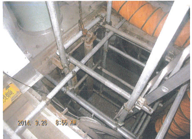
②The customer prepared a foothold near the water surface. Confirmed the repair range is 1.5m
